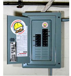
Electrical panel (example)
